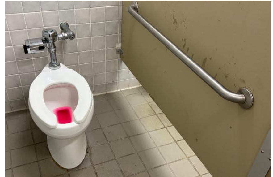
Men's stall with significant signs of wear, undersized space.
