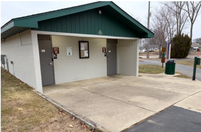
Front of Restroom looking west, aged, cracked concrete, deteriorating retaining wall timbers.
