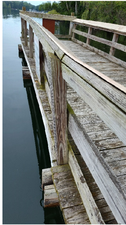
Detached post - lateral deflection
