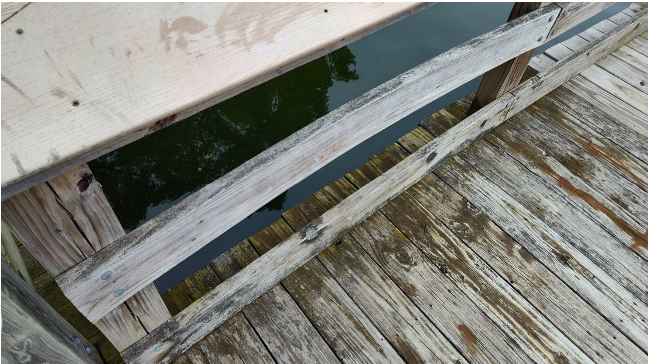
Warped railing board on north pier end
