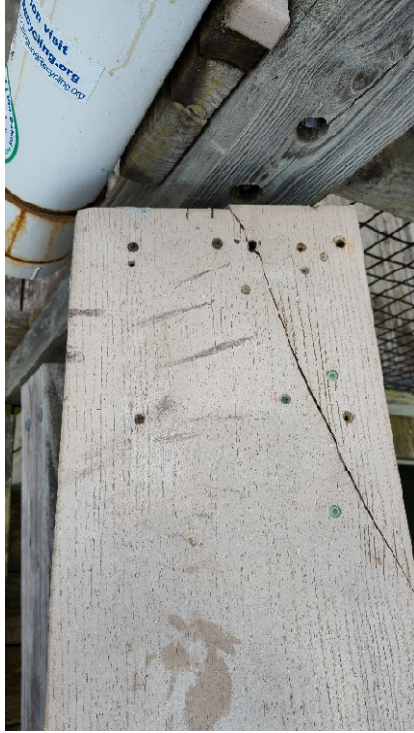
Cracked wearing board on north pier end
