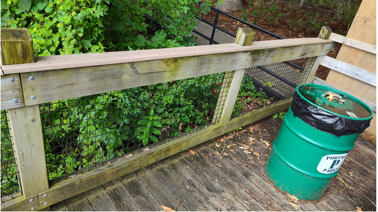
Encroaching vegetation, organic growth, and debris on structure
