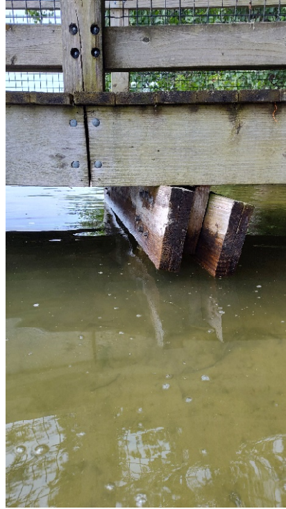
Laterally shifted pile and header
