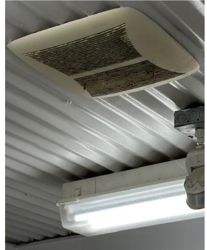
Aged ceiling vents
