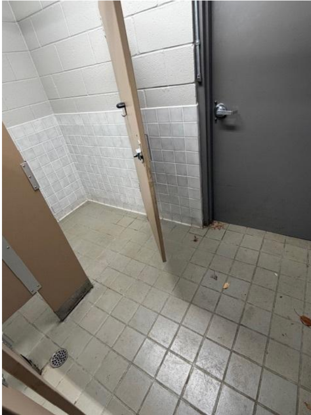
Women's stall door interferes with patrons using entrance door - space is undersized.
