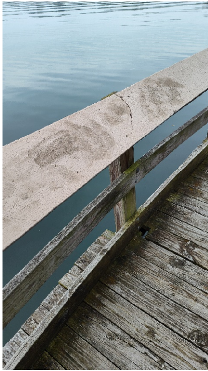
Cracked wearing board at detached post
