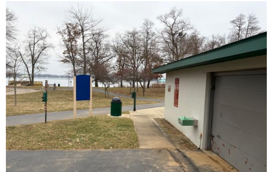
North side of restroom looking east to lake, cracked paved area, rusting door.
