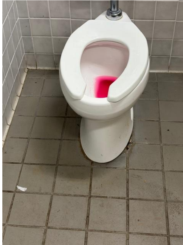
Signs of significant wear, small stall space (not ADA compliant).
