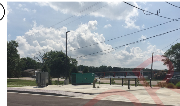
An existing lift station at the corner of Portage Road and Emily Drive represents critical infrastructure, but also presents a physical barrier.
