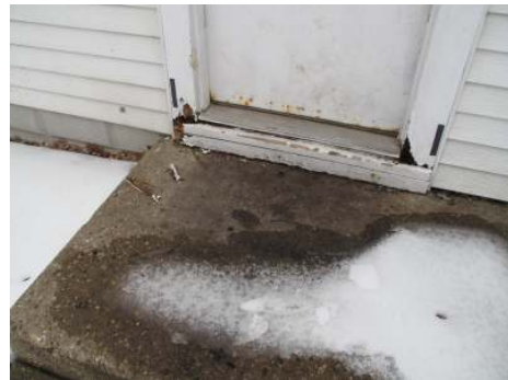
Deteriorating Door Surrounding
