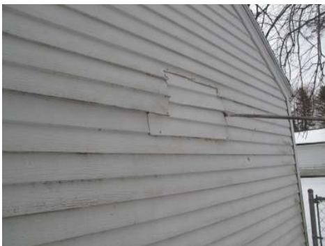
Garage - Former Window (patch)
