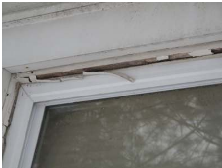
Deteriorating Window Chaulk
