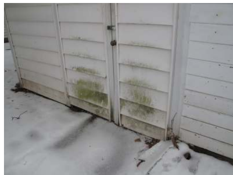
Shed - Possible Mold/Mildew
