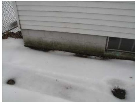
Mold/Mildew on Foundation
