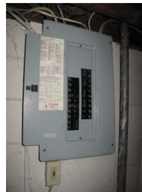
Electrical Circuit Breaker
