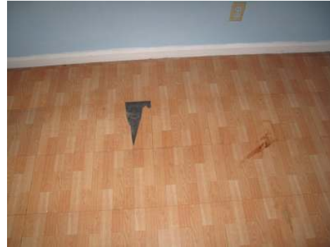
Bedroom #2 - Flooring Damage
