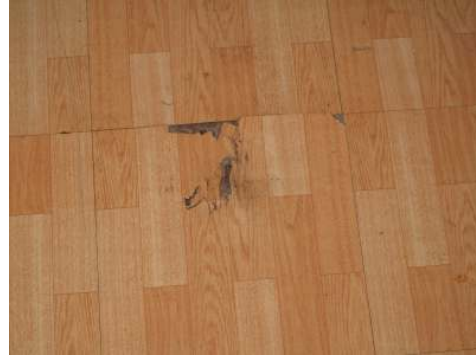
Bedroom #3 - Flooring Damage
