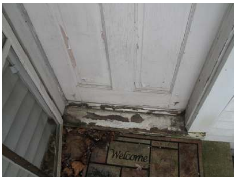
Front Entry Door Needs Painting
