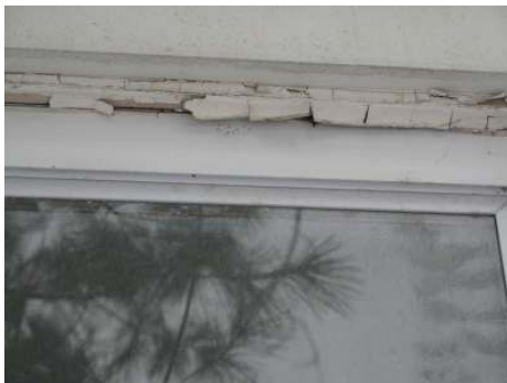
Deteriorating Window Chaulk
