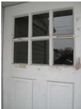
Front Entry Door Needs Painting
