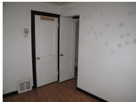
Bedroom #3 - Wall Needs Painting
