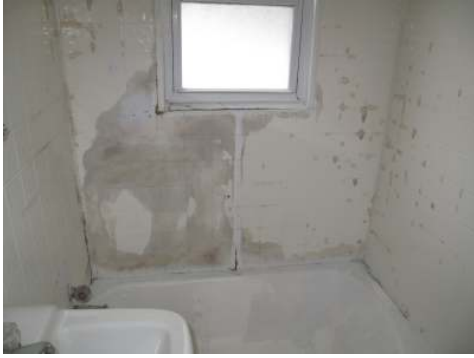
Bath - Wall Damage
