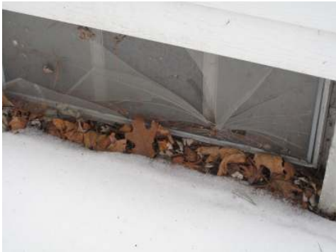
Broken Basement Window
