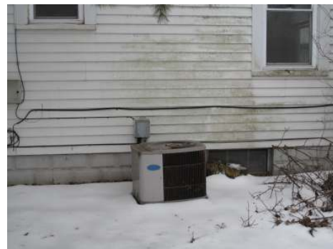
Air Conditioning/Mold-Mildew on Siding
