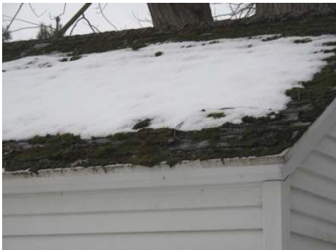
Garage - Heavy Moss on Roof Shingles
